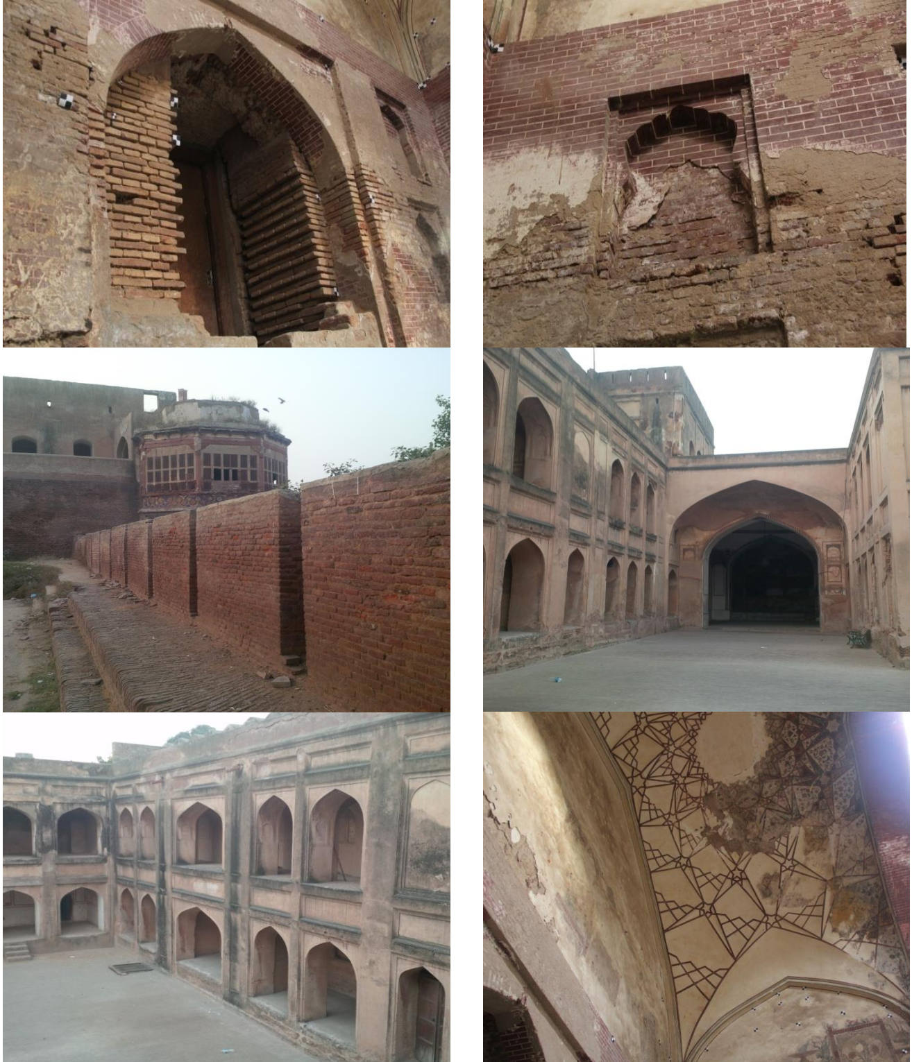
Figure 1: Historical buildings deterioration with the use of cement at different locations for repairs
