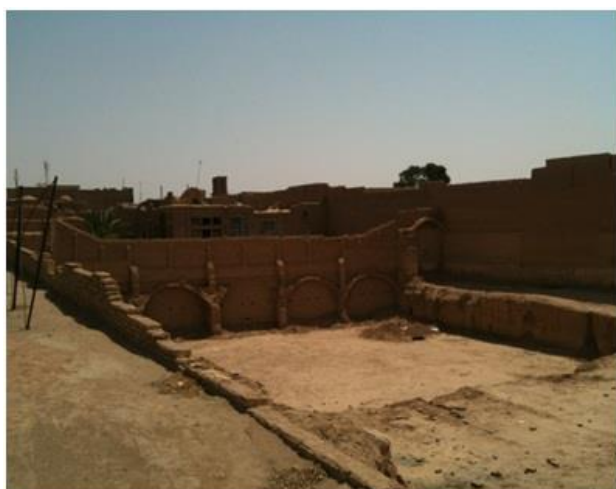
Figure 12. The remaining of demolished historical buildings and monuments on the façade of Basij Boulevard. Source: Authors own construct.
