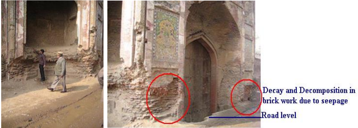
Figure – 10: Picture showing the northern main gate of Shalimar Garden. The levels of the surrounding road is higher than the natural ground level of the garden, causing water ingress in the foundations.
