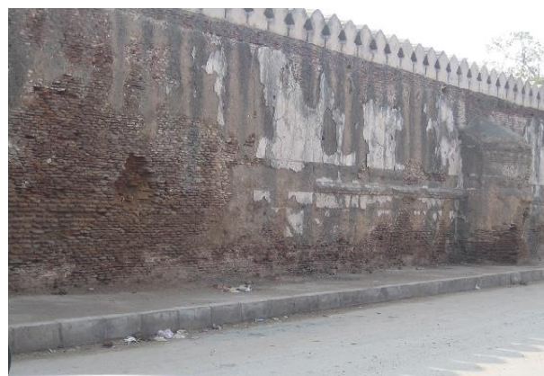
Figure – 18: Picture showing Eastern wall of Shalimar Garden, which shows a bad workmanship and improper restoration during maintenance of the wall in the past. Aesthetic look has not been taken into account during restoration process which gives a adverse impact to the viewers/visitors.
