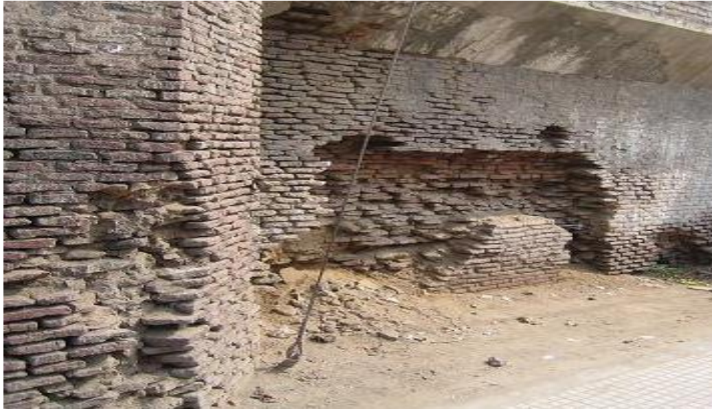
Figure – 8: Pictures showing decay in the northern walls of Shalimar Garden. Photographs were taken on 08-02-2008
