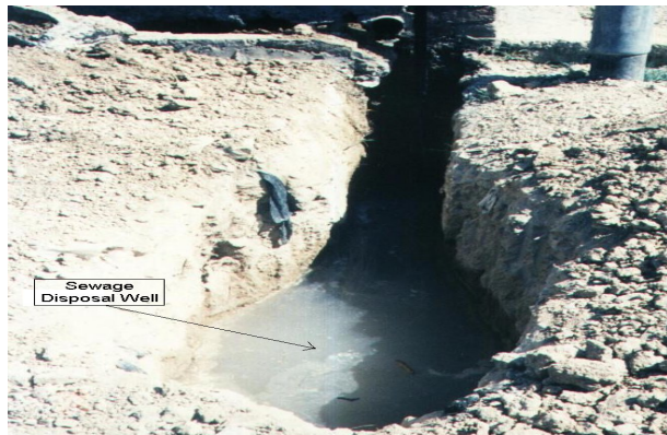
Fig. 2 Sewage disposal well in hard rock containing shallow aquifer in Gulshan colony.
